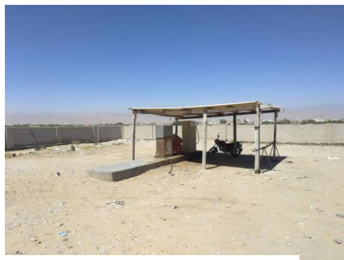
Deteriorated petrol pump for refueling fishing boats
