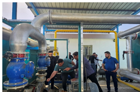
O&M CDAs visited Al-Somoud Water Complex in Albo-Manea Area to discuss operational challenges and identify maintenance issues, such as chlorination devices, horizontal pumps, air-conditioning split units, and an RO filter. UNDP Engineers and O&M provided expertise to address these issues, equipping operators with knowledge and skills for periodic maintenance.
