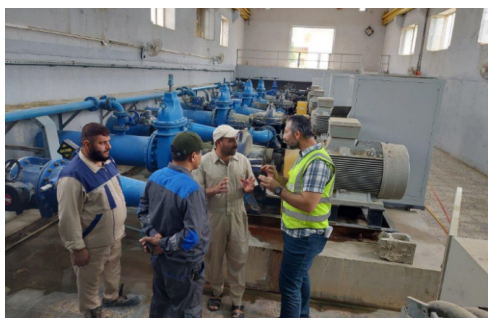
O&M/CDAs visited the Al-Bakr water treatment plant, which operates at a capacity of 500 cubic meters per hour, and delivered a session on the types of water treatment plants and the operating principles for each type.
