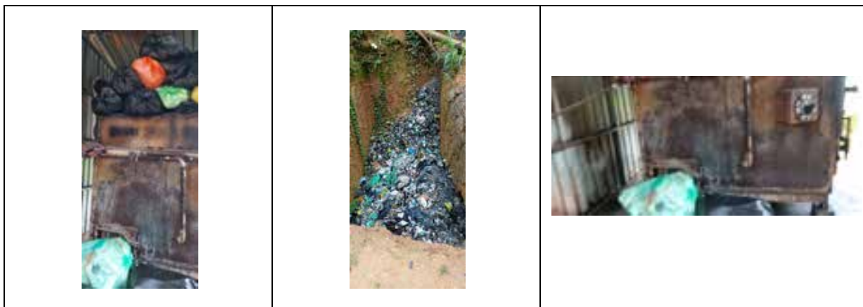
Damaged incinerator due to a fire
