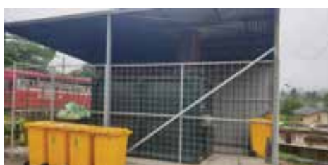
New Incinerator in Badulla Hospital
