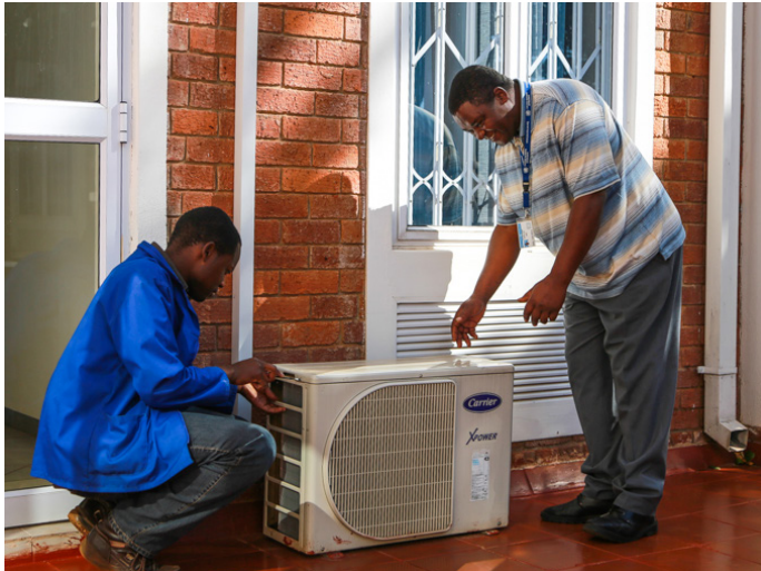
Yusuf Size (right) working with Simbarashe (left) to de-commission the older generation of air conditioning units which used a lot of energy.
